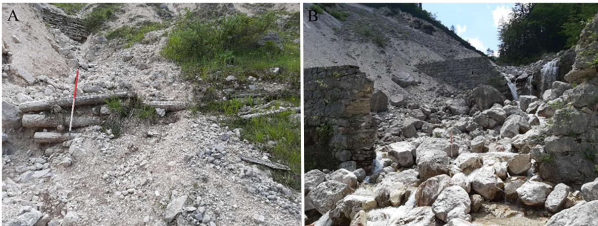
Figure 32. Completely destroyed torrent control measures that provide no protective function. Location: Kranjska Gora. (Photo: Domen Oven).
