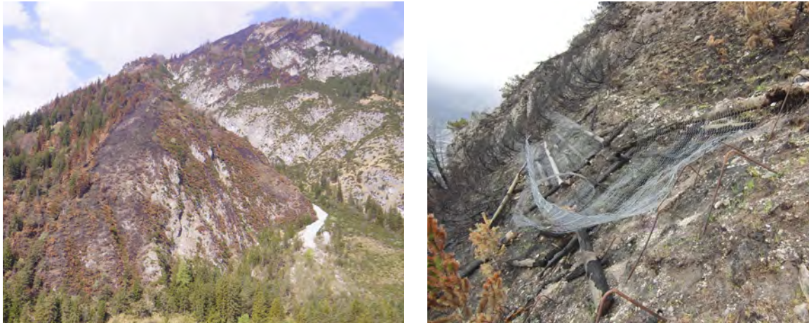
Figure 21 Overview of lower burnt section at the Hochmahdkopf on 24 April 2014 (left); damaged avalanche defense structures and charred mountain pine in the upper burnt section on 10 April 2014 (right).
